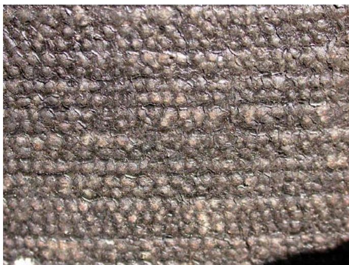
Figure 1 – Photo showing typical as-cast peen pattern surface on DI Pipe
