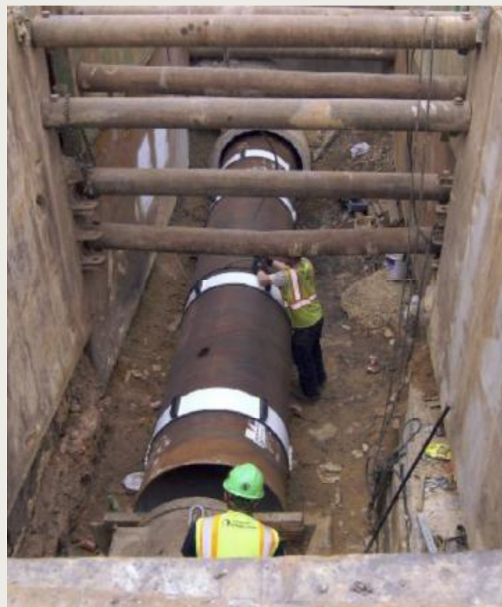
After failing a couple of times, the 48-inch Kenilworth Transmission Main in Baltimore County, Maryland, underwent a permanent structural rehabilitation using steel pipe sliplining.
