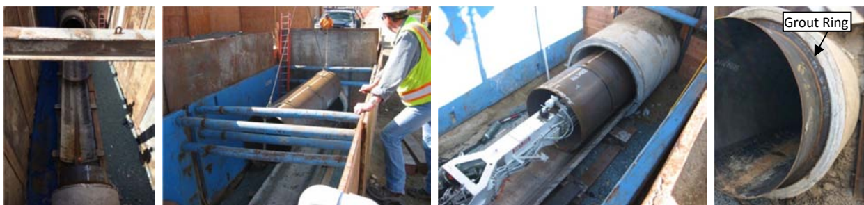
Figures 9a, b, c, d: Portal with 2 Sections of Host PCCP Removed, Steel Reliner being Lowered into Portal, Insertion of Reliner Section into Host Line on Pipe Carrier Cart, Installed Grout Ring
