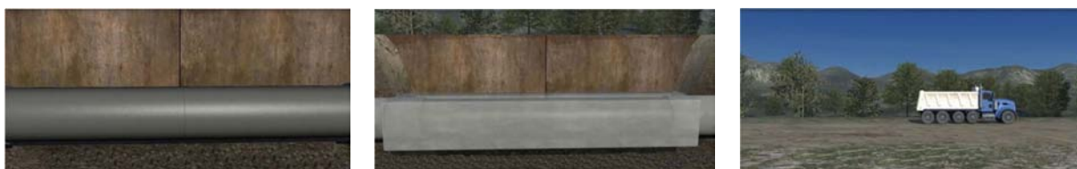
Figures 3a, b, c: New Steel Pipe Sections Placed at Portal where 2 Sections of PCCP was Removed, Reinforced Steel and Concrete around New Pipe, Portal Backfilled
