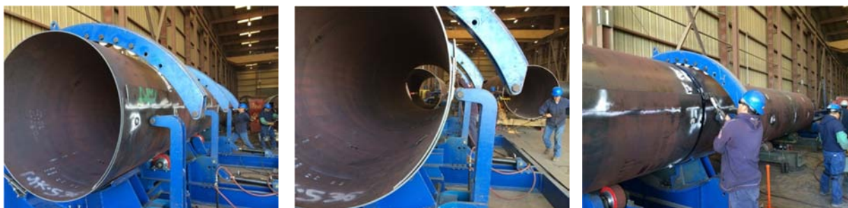
Figures 7a, b, c: New Steel Pipe Sections Placed at Portal where 2 Sections of PCCP was Removed, Reinforced Steel and Concrete around New Pipe, Portal Backfilled
