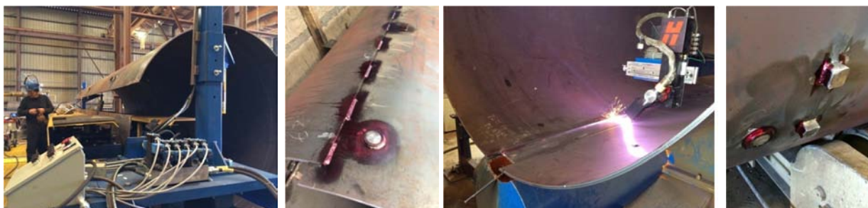
Figures 6a, b, c, d: Preparation for Backup Bar Forming, Completed Backup-Bar with Dye-Penetrant Testing Complete, Stitch Cutting of Backup Bar Prior to Collapsing, Dye-Penetrant Testing of Welded Spacer Blocks and Grout Couplings
