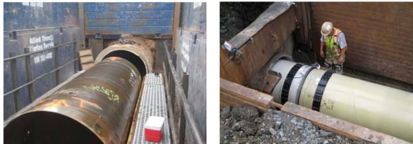
Figure 2a, b: Sliplining 60-inch PCCP in Phoenix, Sliplining 48-inch PCCP in Halifax, Nova Scotia (Bass 2011)
