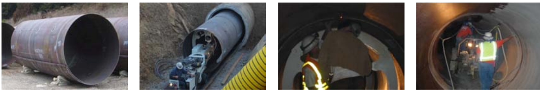
Figure 1a, b, c, d: Collapsed Reliner Cylinder, Insertion of Reliner into Host PCCP, Expansion and Welding of Reliner, In-field Lining Application
