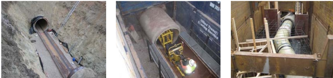
Figure 4a, b, c: Insertion Portal for 96-in Dia. PCCP at SDCWA, 60-in Dia. PCCP Portal in Highly Urban Section of City of Phoenix, Insertion Portal for 48-inch PCCP at a Bend in Halifax, Nova Scotia
