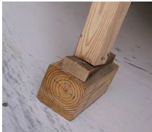
Figure 16: Support feet at the end of each stull
