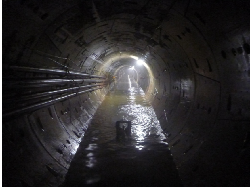
Figure 11. Flooded Tunnel at 2 nd Dip.
