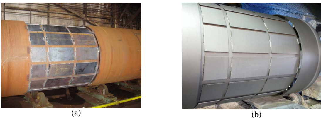
Figure 1. Pipe with smaller diameter section to accommodate flat panels for the cleaning and coating processes (a) prior to blasting, (b) after blasting.
